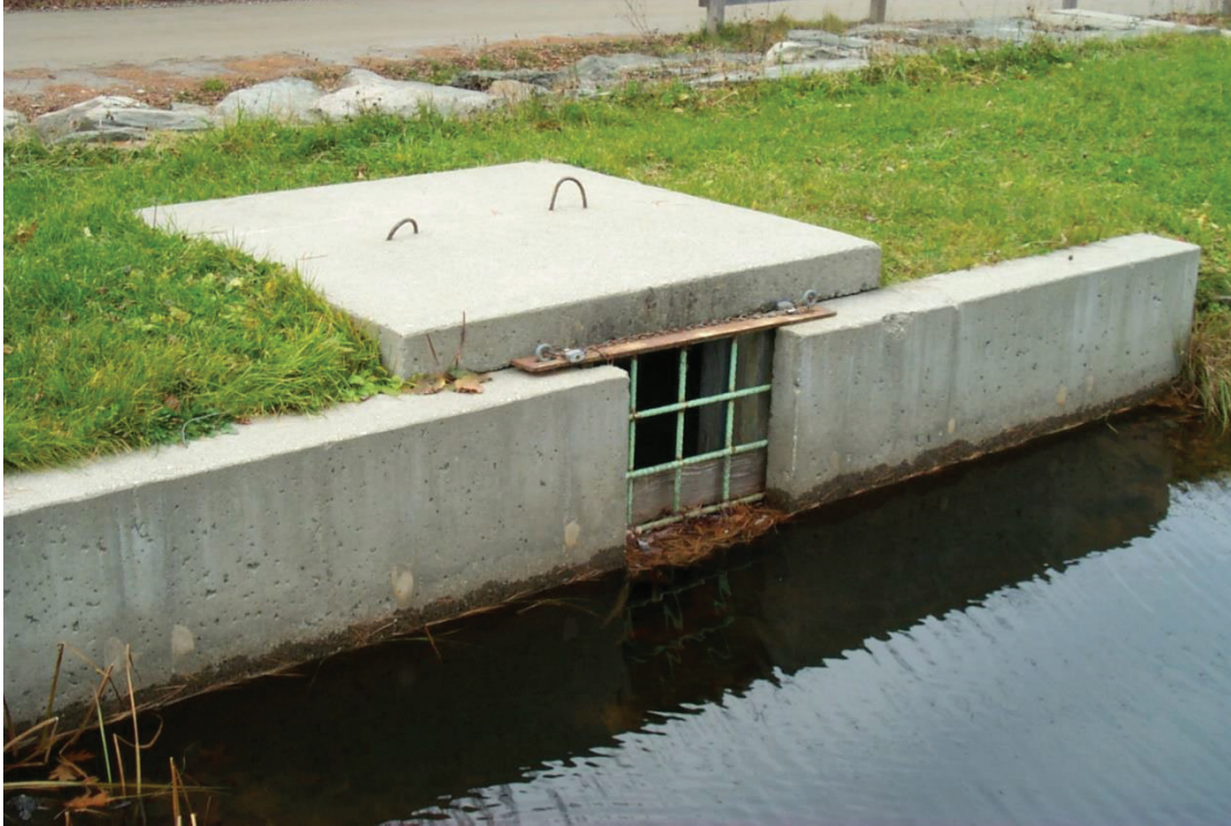
Figure C-9 - Photo dated 11/7/2000 of the pond drain at the left end of the Lake Warren Dam showing the boards that control flow through the pond drain.
