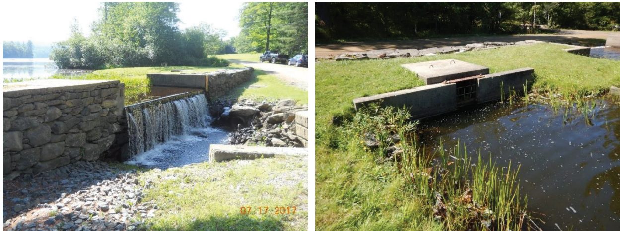
Figure C-6 - Lake Warren Dam spillway from downstream (7/17/2017) and the pond drain structure with the spillway in the background (9/13/2019)
